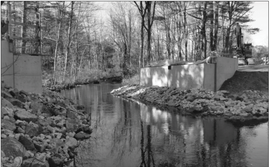
New bridge abutments at the Nute Road Bridge over the Bellamy River.
