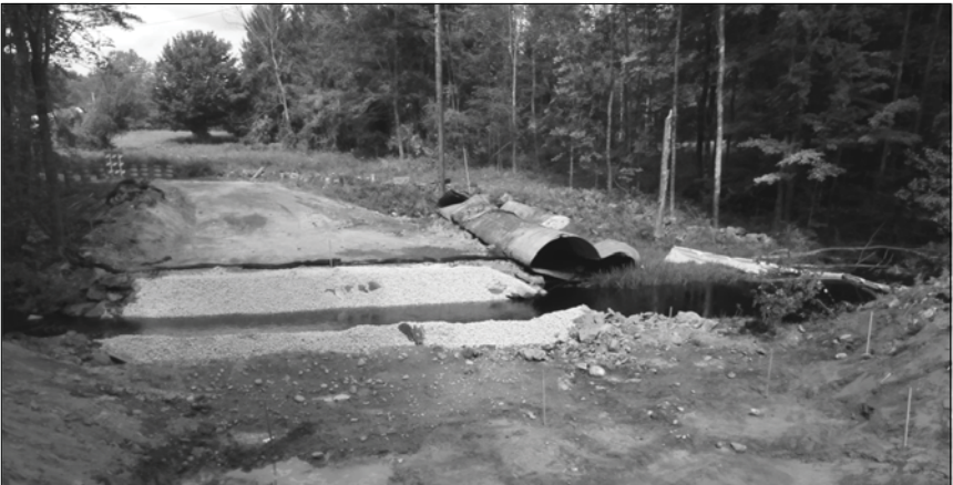
Old Nute Road Bridge is gone.
